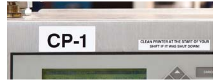
Control Panel & Electrical Panel Labels
